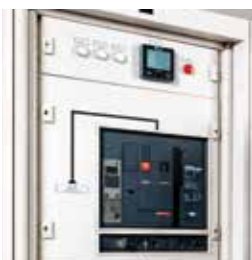
Main LV switchboard
